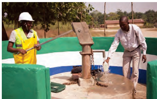
Water pump installation
